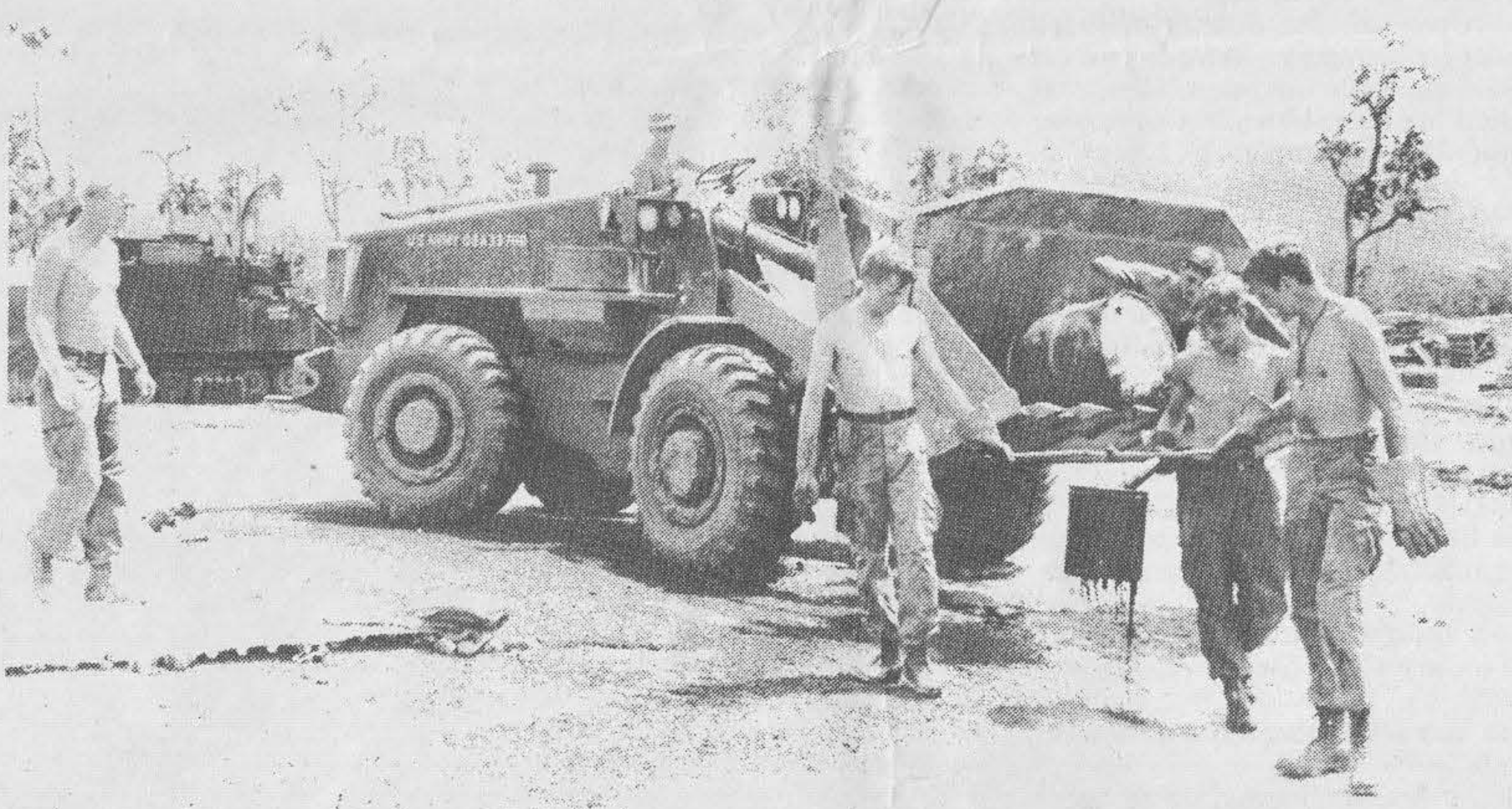
Those oily "Red Devils" with their funny looking machine -- 919th Engineers put down penta-prime on the pad at Fire Support Base Bolan.
